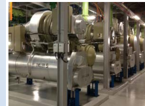
Optimising Air-conditioning Plant
